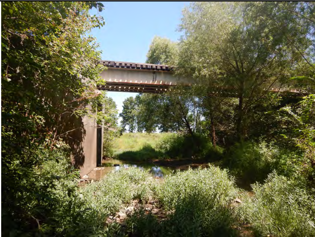
Photo 14: View of the crossing over Inola Creek from the south side of the bridge. Facing north.
